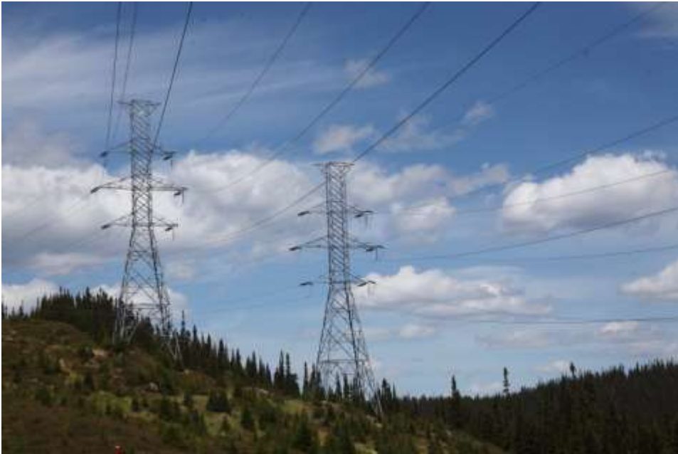
High tension electrical transmission towers and lines
