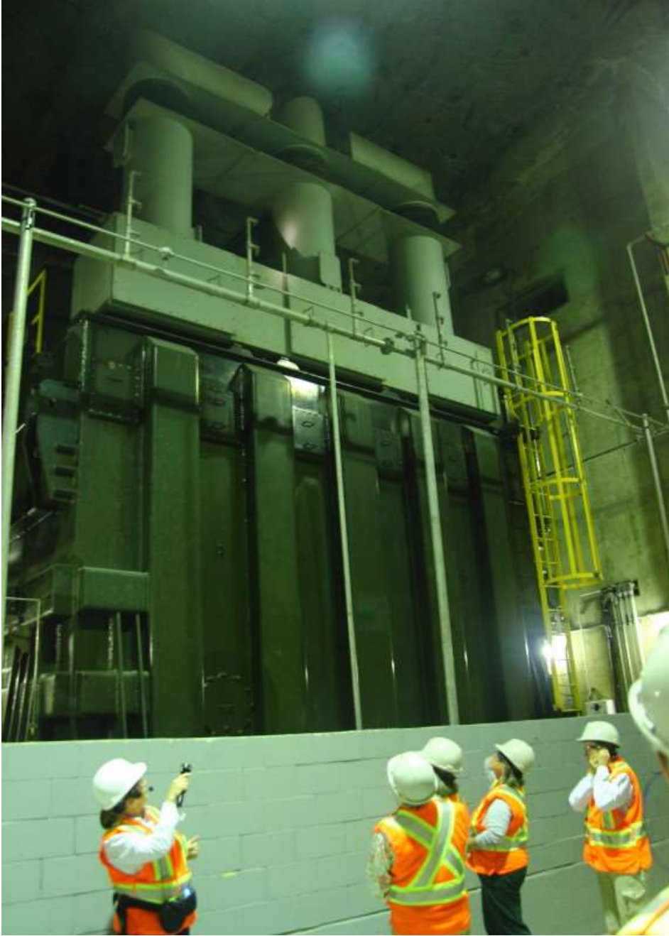
One of 11 transformers
