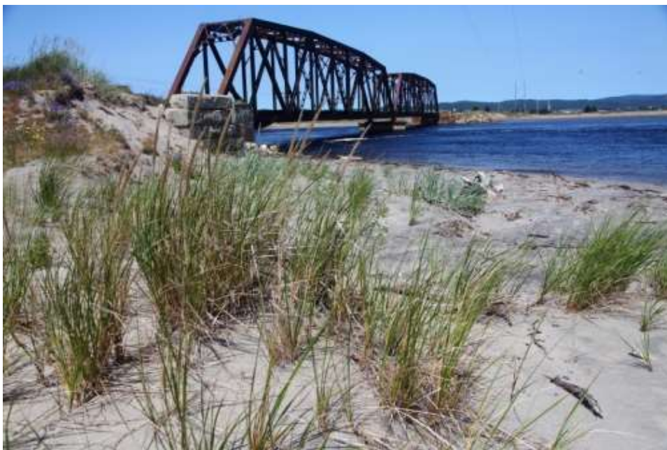
Dilapidated bridge near Stephenville
