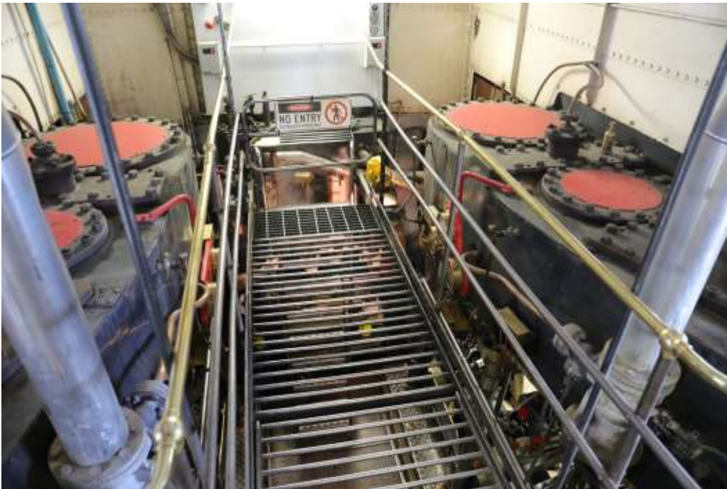
Steamship boiler room of TSS Earnslaw
