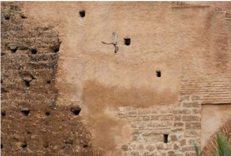
Chellah wall with square holes used for scaffolding during construction and air passage later
